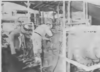
Mechanical-Trade man "A" - mechanists Guillermo Yarzagaray (l) and Bibiano Lopez (r) get assistance from Alfred Schaeferling (c), of AEG-Kenis during assembly of turbine driver for Hydrogen compressor.
